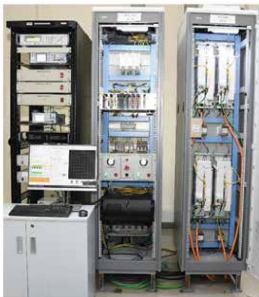
Servo Control System
