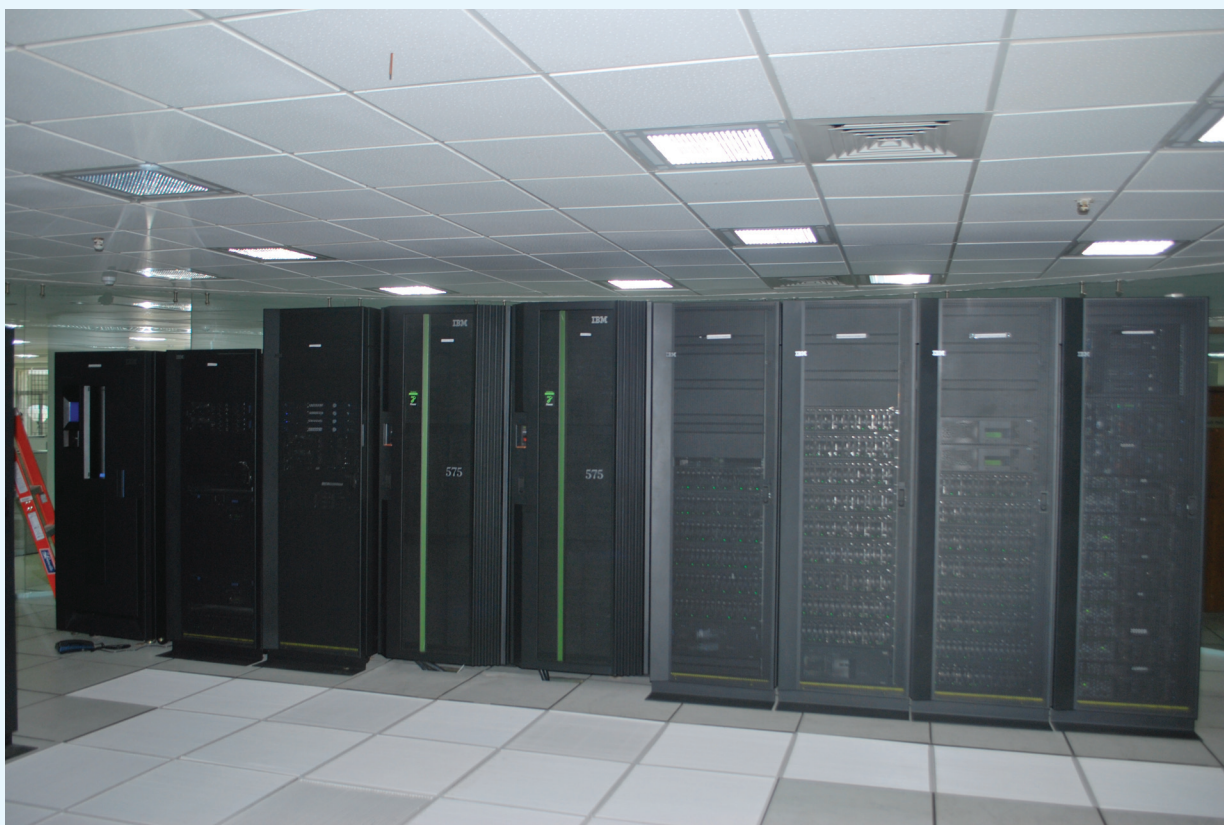
HPC facility at INCOIS
